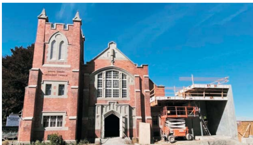
The Ashburton Methodist Parish Baring Square Church requires a new roof in addition to planned renovations.
