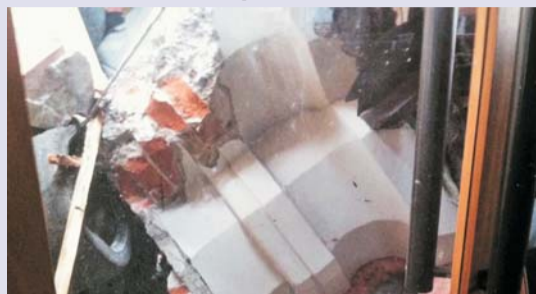
Church roof collapses
