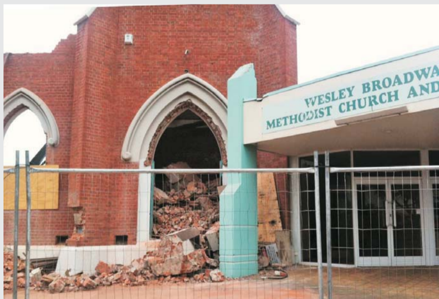
Demolition was underway when an unexpected chunk of masonry fell into the church foyer.
