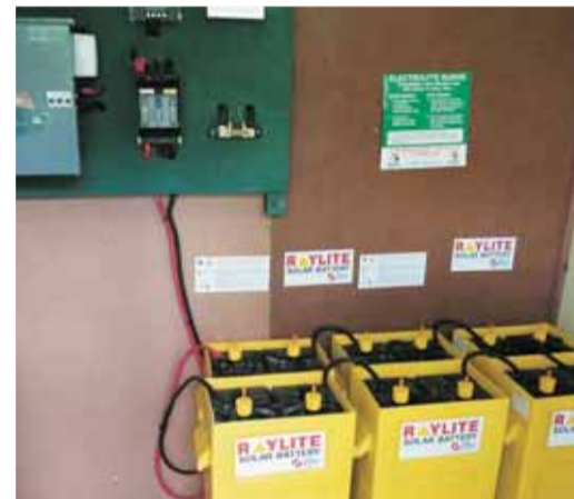
The solar power system freshly installed at Sasamuqa Hospital.
