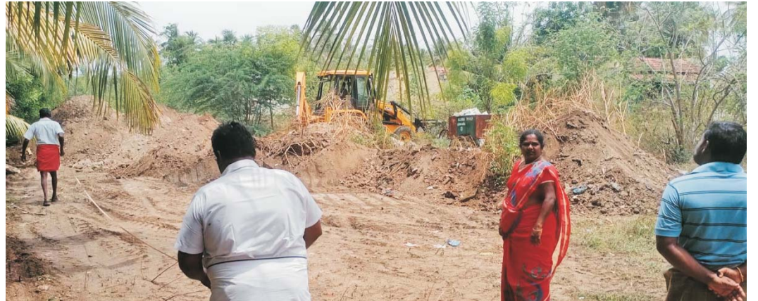
Newly elected Panchayat or local council president, Senthamarai has taken up the challenge of protecting eight villages from hunger and Covid-19 in badly affected Tamil Nadu, India. Here she supervises the digging of a new well so villagers have clean water. Credit: HRF.
