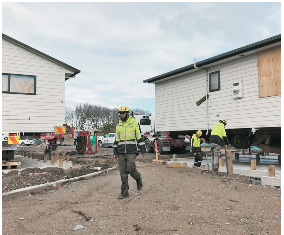
The first two of 16 homes at CMM's new housing development being lowered onto foundations.
