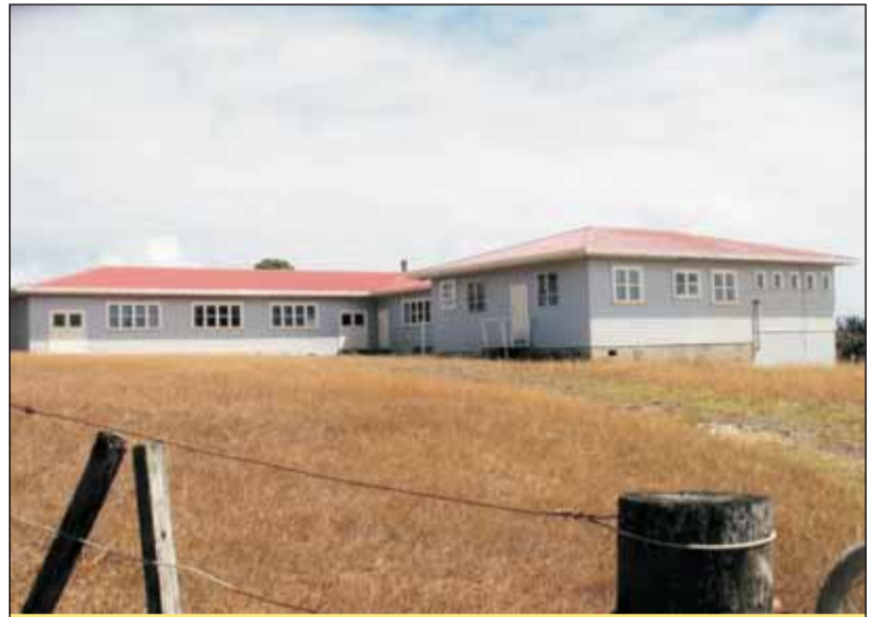
Thanks to the work of volunteers and financial support from the Church, Red Hill Camp now has a new roof.
