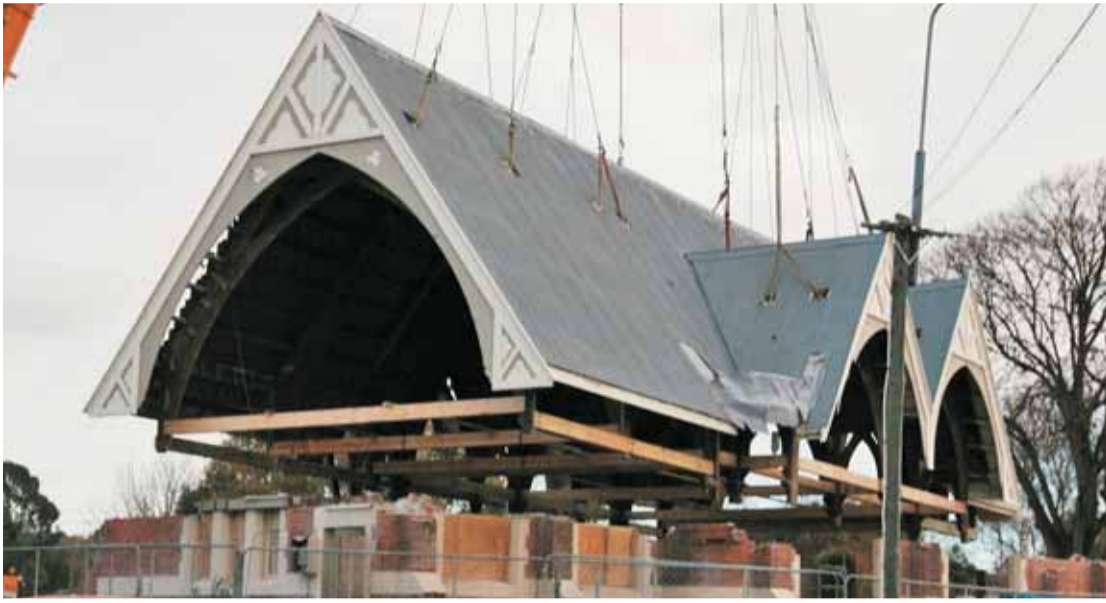
The old roof of Opawa Methodist Church will sit on a new building.
