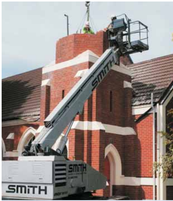
Earthquake-damaged Papanui Methodist Church will be farewelled on Nov 30th
