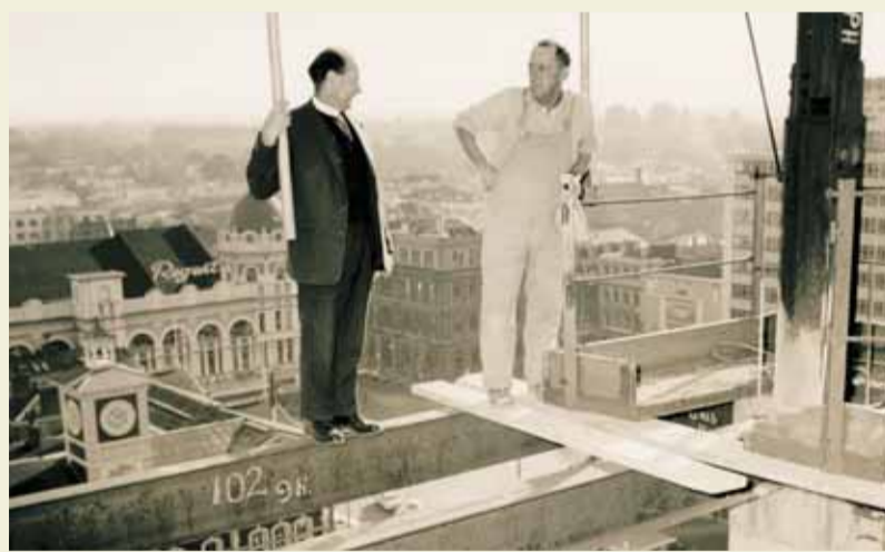
Rev KA Hadfield standing on a steel girder overlooking Christchurch's Cathedral Square during the construction of the Bank of New Zealand building, 1966.
