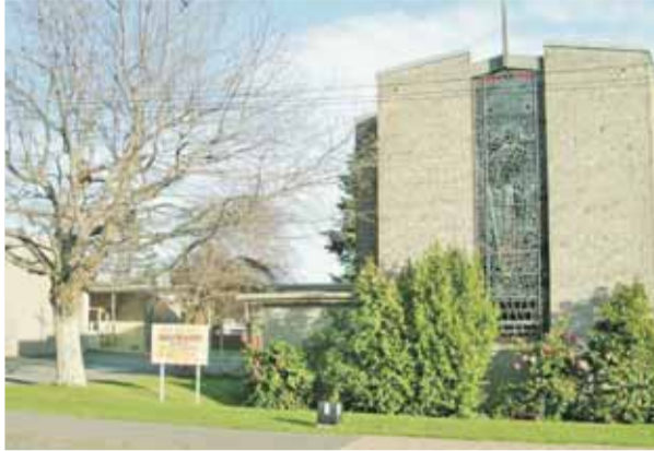
Most of Stoke Methodist Church's buildings are off-limits, and the congregation is finding ways to link up with other local churches.
