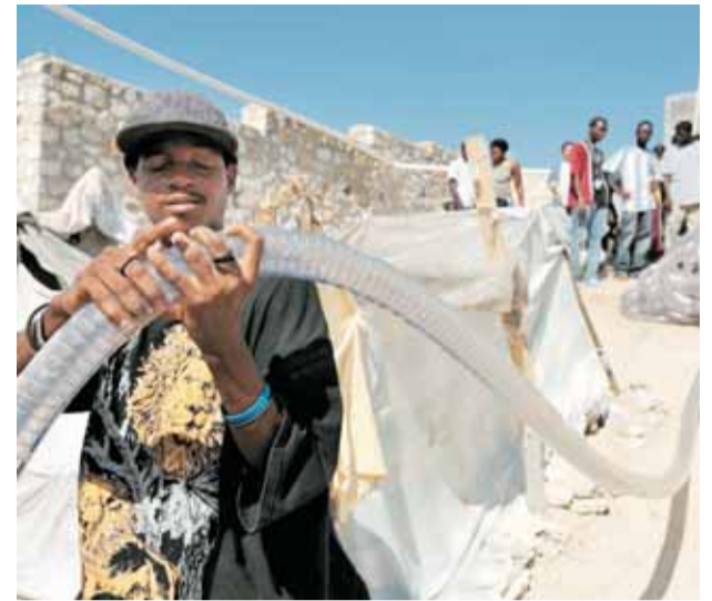
Emergency workers from ACT Alliance unroll piping for safe water supplies soon after the quake. Systems such as these helped avoid outbreaks of disease.
