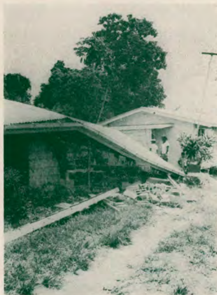
Damaged buildings at Gaulim Teachers' College.
