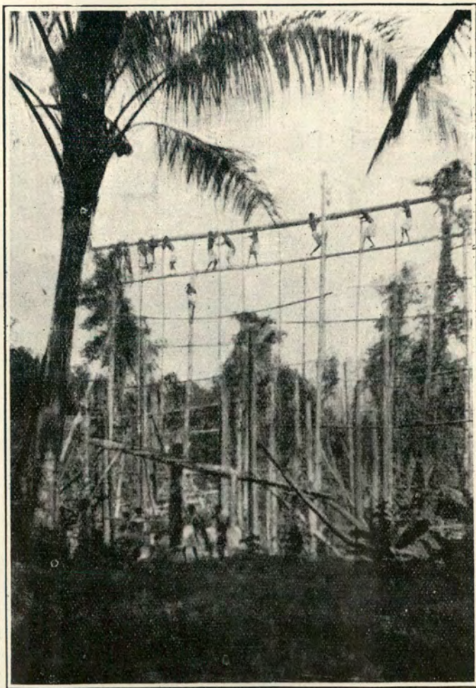
Building a Church on Choiseul by the natives. The ridge-pole being lashed in position. Photo: Rev. V. le C. Binet.
