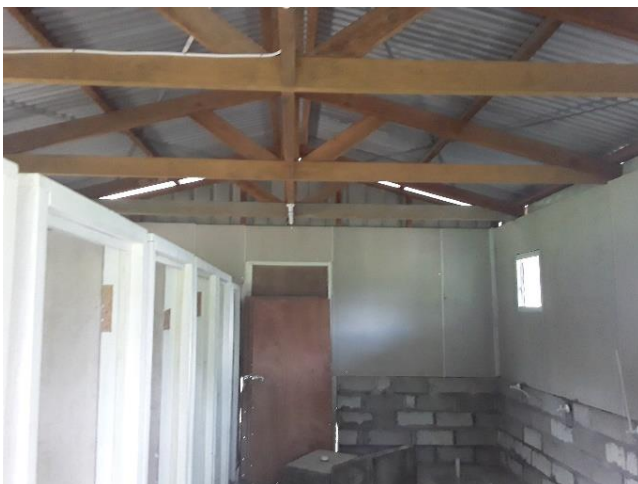
The interior of the Ablution and Shower facility under construction at the Tabaka Rural Technical Institute
