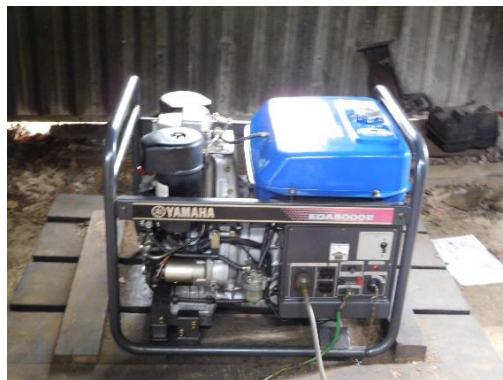
The diesel generator provided by M&E is in full use
