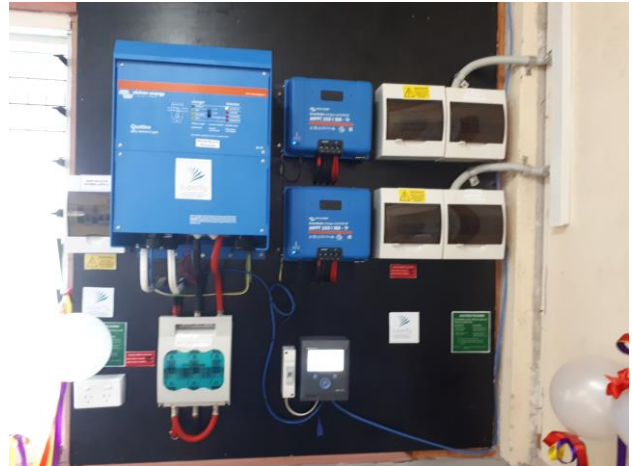
The Power distribution centre of the computer lab
